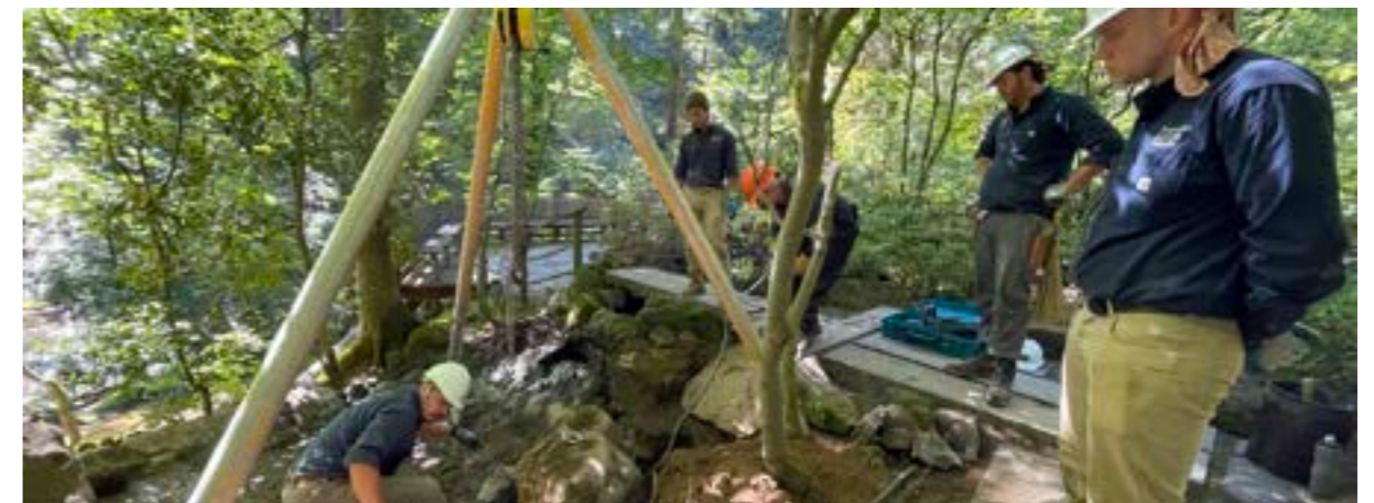
Garden Curator Hugo Torii and his team in the Garden Department getting ready to move massive boulders out of the way as they repair this part of the Natural Garden.
